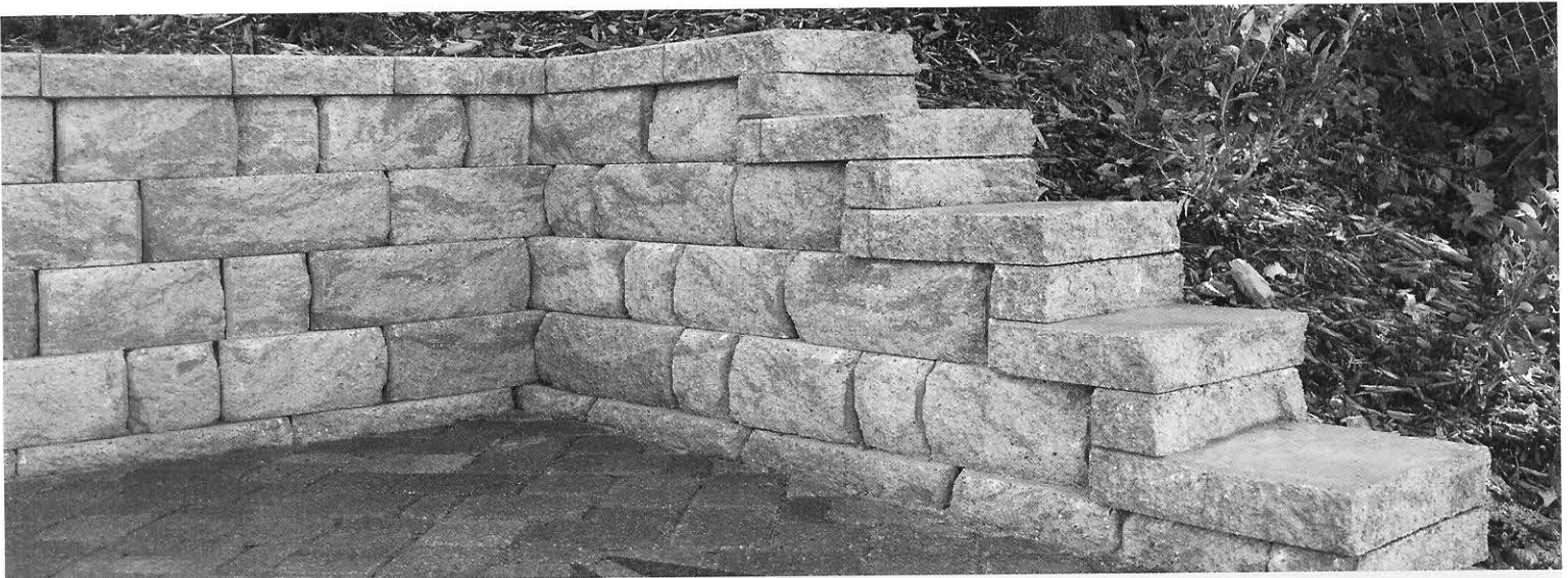
A quiet corner is sheltered with an inside 90° corner built with Highland Stone.® Step up the caps in 3-inch increments for a finished look. See page 24 for more information about stepping up caps.
